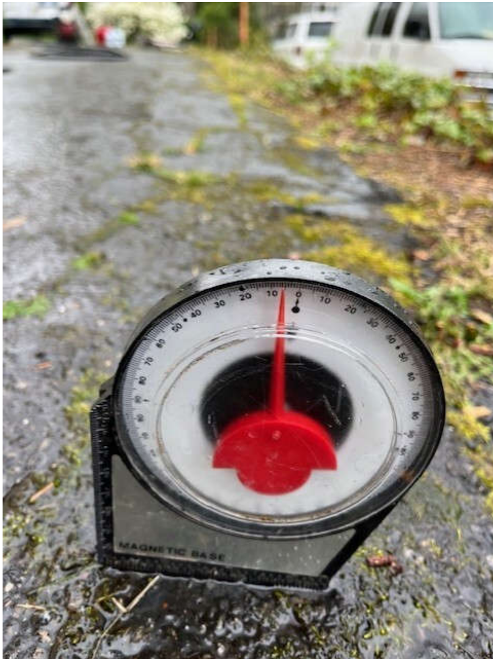
Photograph 4: Sloping at distressed portion of driveway.
