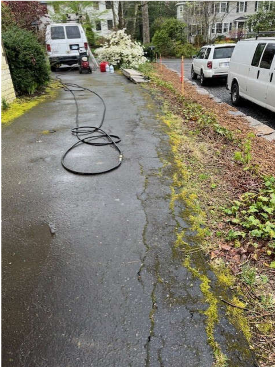
Photograph 4: Cracking at outside edge of asphalt driveway. Widman residence on left.
