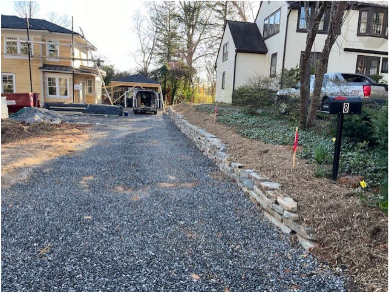
Photograph 3: Property boundary viewed from White Oak Road, looking east, showing new retaining wall. Widman residence on right.
